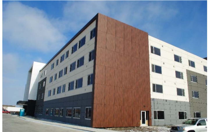
Over 10,000 sq. ft. of RevealShield SA Self-Adhered Black, UV Stable Water Resistive Vapor Permeable Air Barrier Membrane was installed behind Trespa Miteon open joint panels on the Element Hotel in Fargo, ND.
